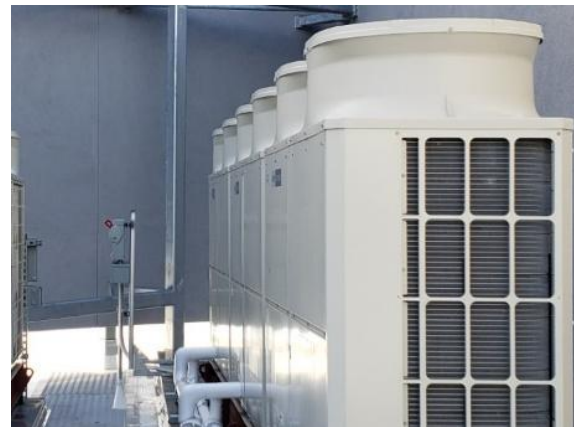
Figure 1: VRF central outdoor compressors
