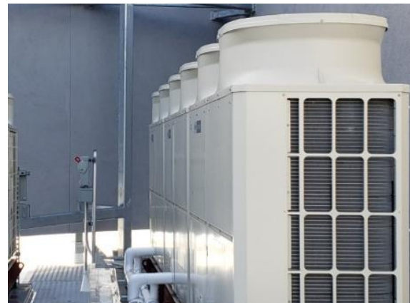
Figure 1: VRF central outdoor compressors
