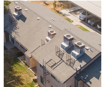
(Below) View of rooftop HVAC units before retrofit.
