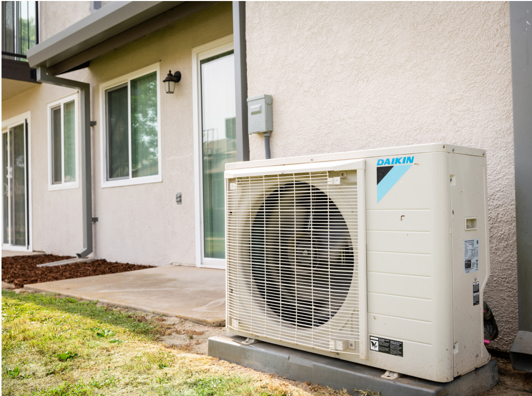
(Left) New heat pump condenser unit after retrofit. This particular heat pump serves Apartment A of Building 615.
