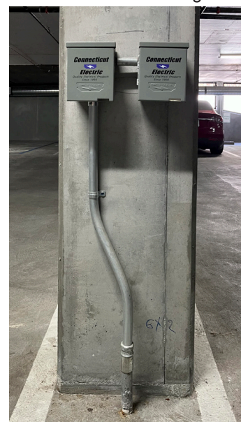
(Below) Electric car charging units in basement Garage.
