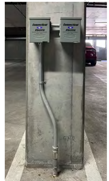
(Below) Electric car charging units in basement Garage.
