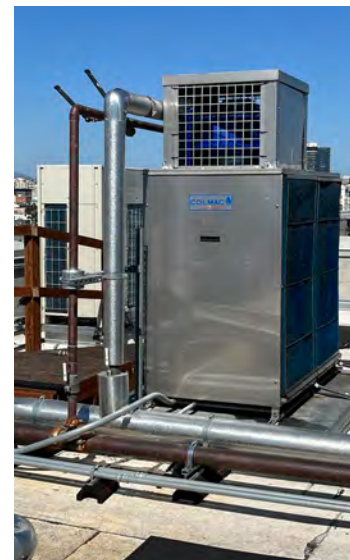
(Above) Heat pump water heater located on the roof.
