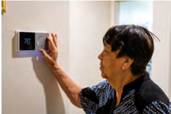
(Above) Retrofits included installation of “smart” thermostats.
