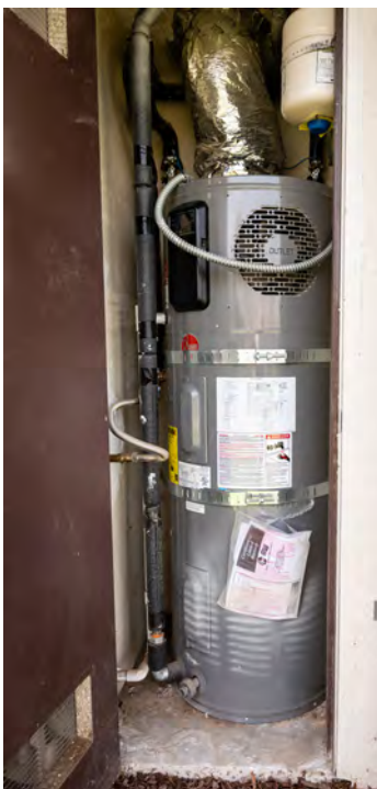
(Below) Packaged heat pump water heaters were located in exterior closets.
