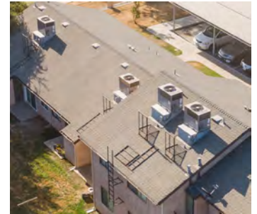
(Below) View of rooftop HVAC units before retrofit.
