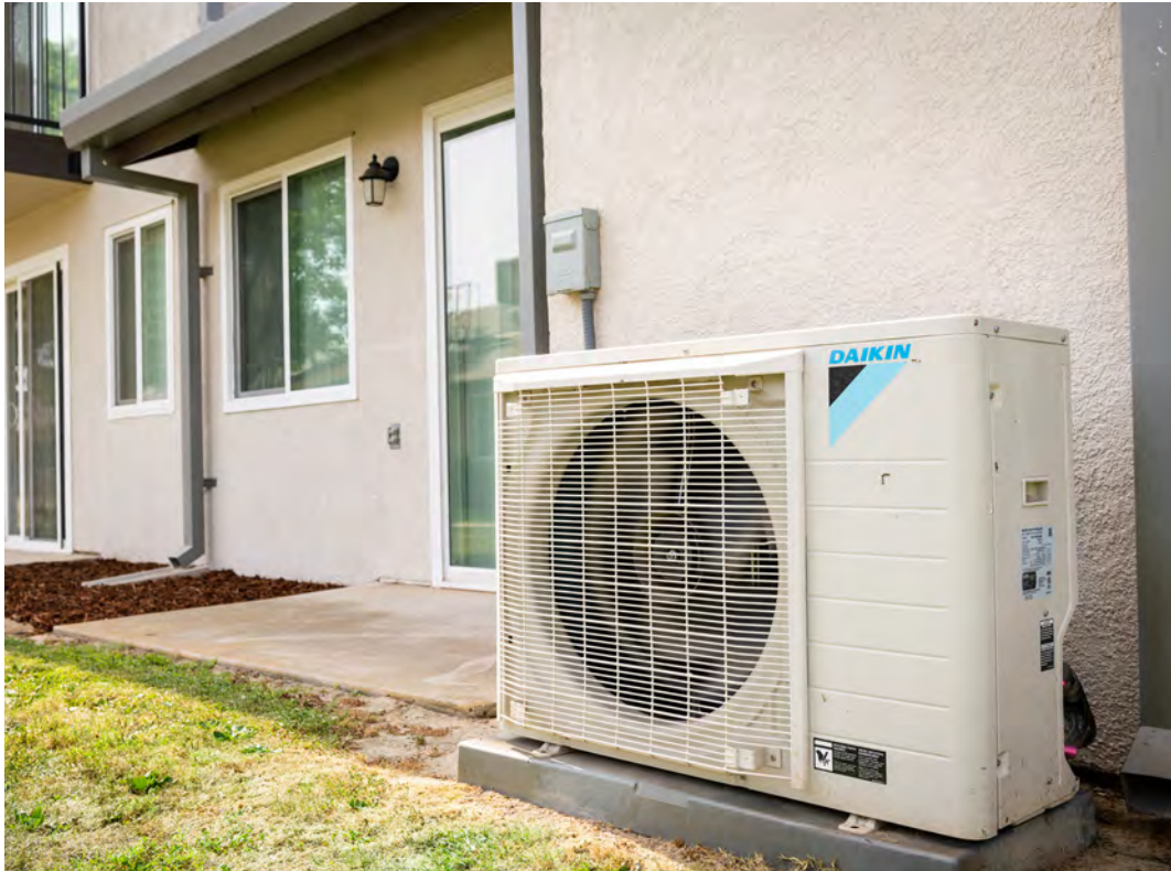
(Left) New heat pump condenser unit after retrofit. This particular heat pump serves Apartment A of Building 615.
