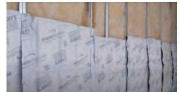
(Above) Phase change material installed over insulation in selective walls. (Courtesy of Buro Happold.)
