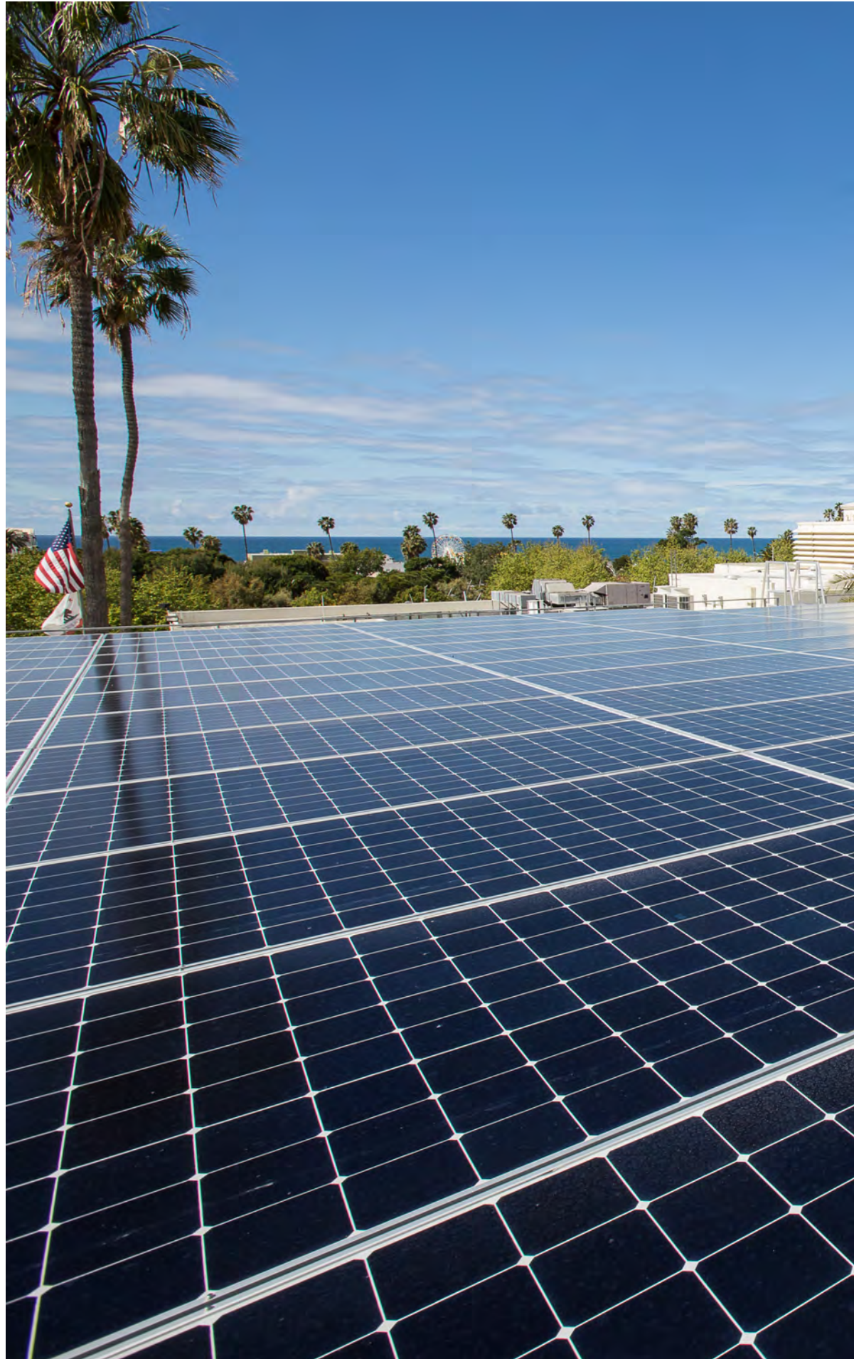
(Right) View over rooftop PV installation toward the north-west and the Pacific Ocean. (Photo: Amy Williams.)
